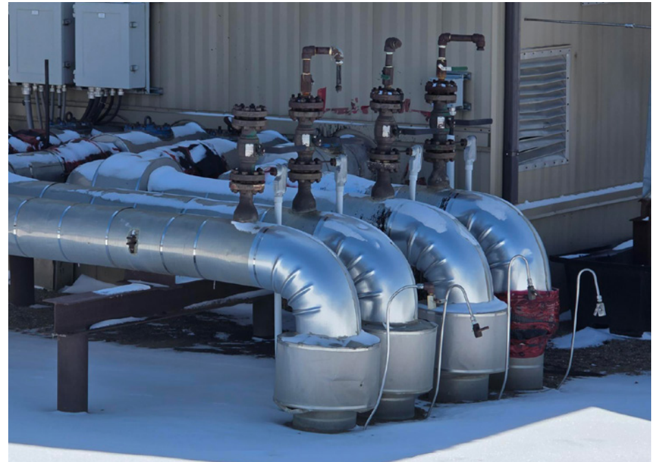
▲ Oil emulsion pipelines at Strathcona's East Bodo facility.
